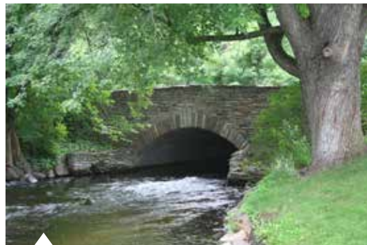
The City has started the design process for rehabilitating or replacing the historic Wooddale Avenue bridge over Minnehaha Creek. File Photo
