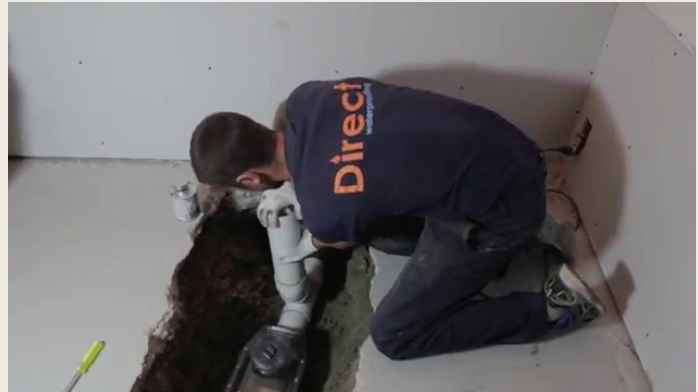
Sanitary backflow preventer installation
