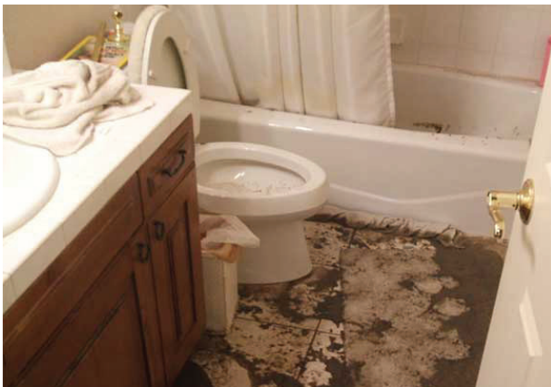
(Top) Image of sewer backup in bathroom, courtesy of https://blueskyplumbingfl.com/wp-content/uploads/2016/10/sewer-backup-in-bathroom.jpg
